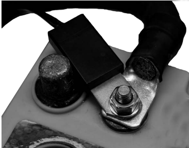
Fig 2.5(b) Temperature Sensor Installation
