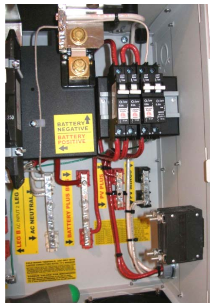
63 amp din rail DC-GFP wired with a 63 amp PV disconnect and a 63 amp controller output breaker.
