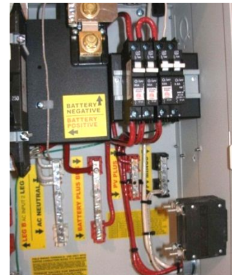
63 amp din rail DC-GFP wired with a 63 amp PV disconnect and a 63 amp controller output breaker.
