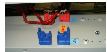
Position new mounting blocks as shown. Secure them with screws removed earlier*
