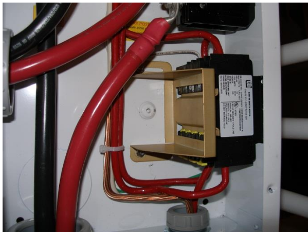
Din Rail mounted breakers
