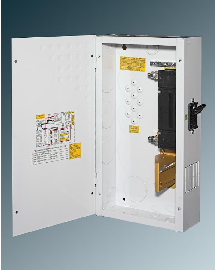
Shown with 250 amp sized breaker
