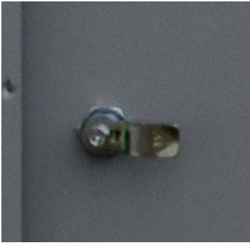
Lock viewed from inside
