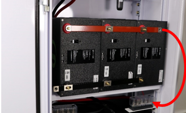
Figure 8.0 - PHI Battery Wiring Using Interconnecting Busbars
